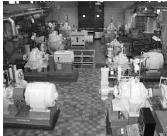
to our Pumping Facility...
