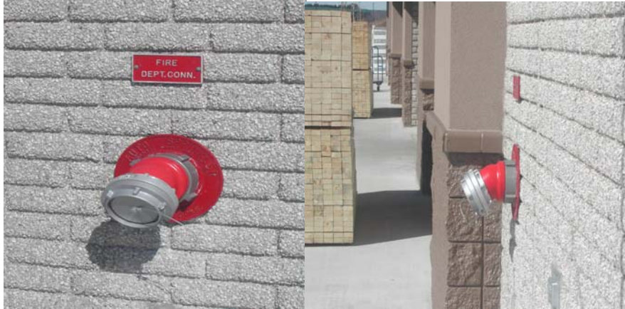
Approved Fire Department Connection
